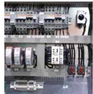
Auto Transfer Switch (ATS)
